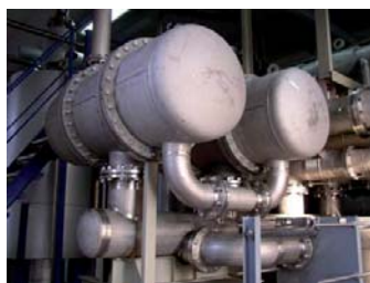
Fig. 2: Installed vapor permeation membrane modules in the demonstration plant
