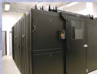
Main data centre room
