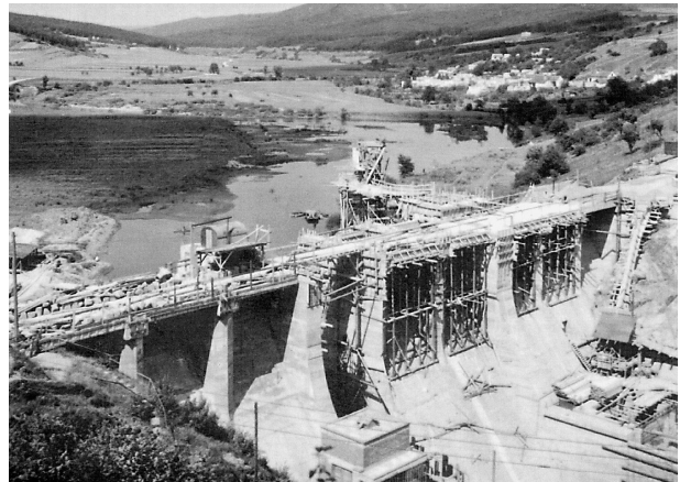
Figure 1: View on the valley and constructed dam (source: Photo Collection 1939, afford by doc. Miroslav Šlezinger – VUT Brno)
