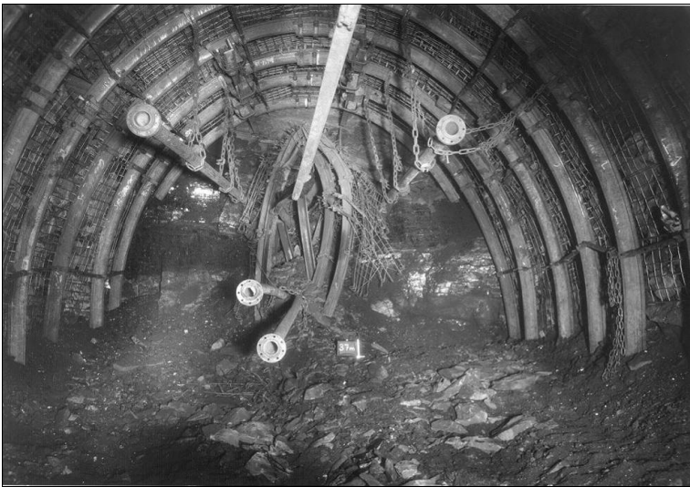
Fig. 1. Rockburst: total destruction of the roadway
