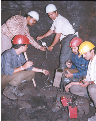
Fig. 9. Installation of a vibrating wire stress meter in a horizontally drilled hole
