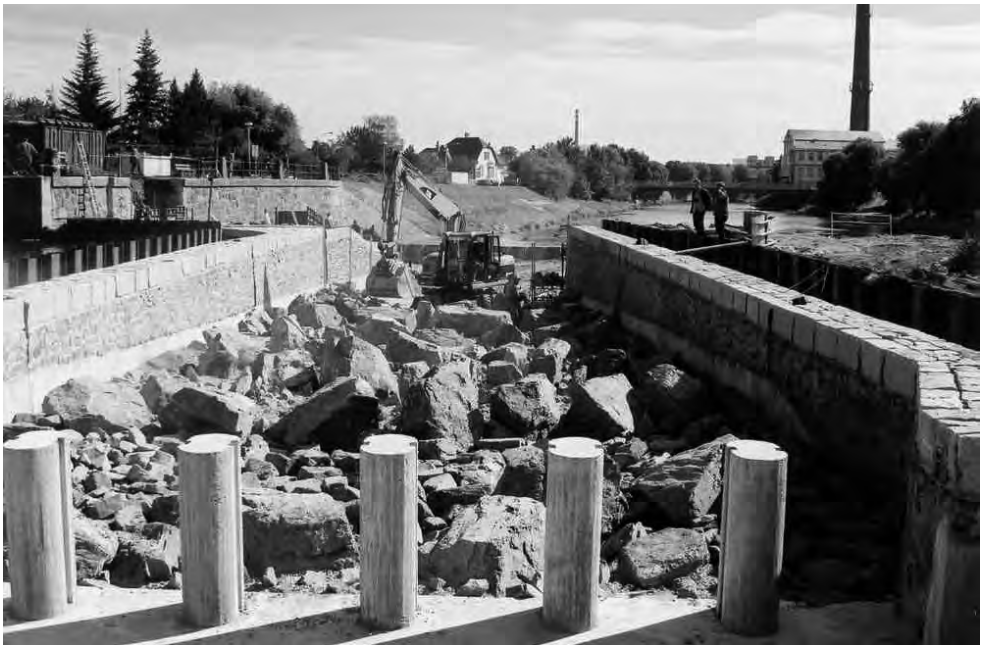
Building of fish pass on the Dyje River in Břeclav. (Photo by K. Halačka)
