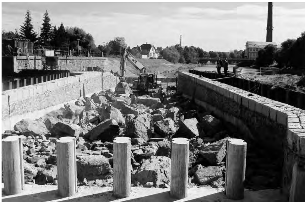
Building of fish pass on the Dyje River in Břeclav. (Photo by K. Halačka)
