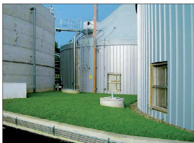
Biogas device (source: Renergy, s.r.o.)
