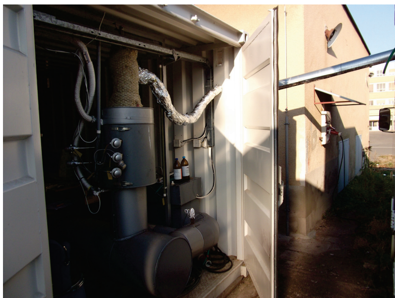
The combined thermal desorption and catalytic oxidation unit
