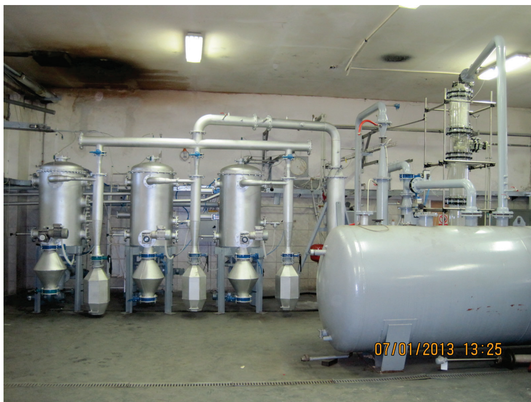
Grateless moving bed gasifiers
