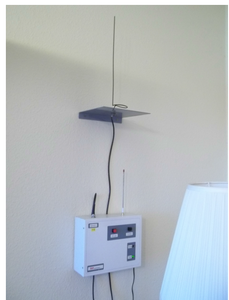
© Emergency Alarm System
