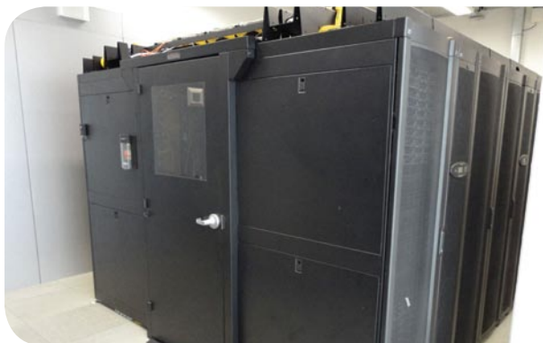
Main data centre room
