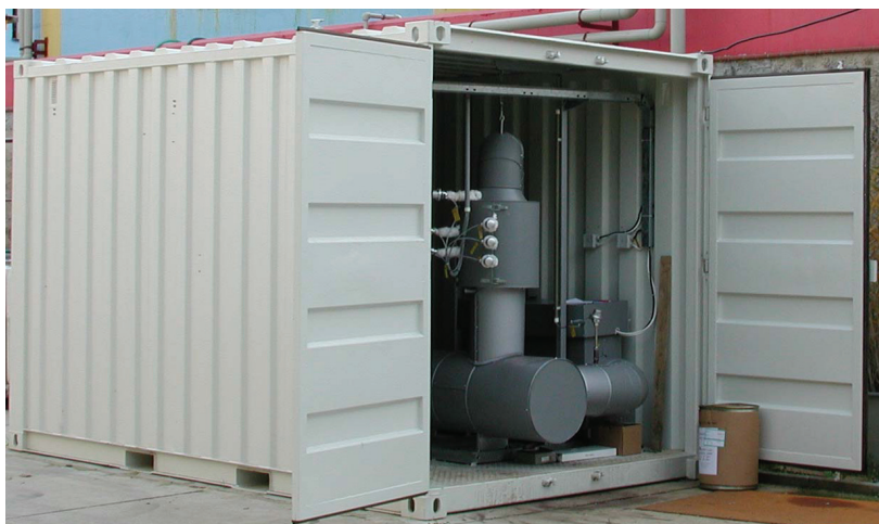
Pilot unit for catalytic oxidation of desorbed organic contaminants
