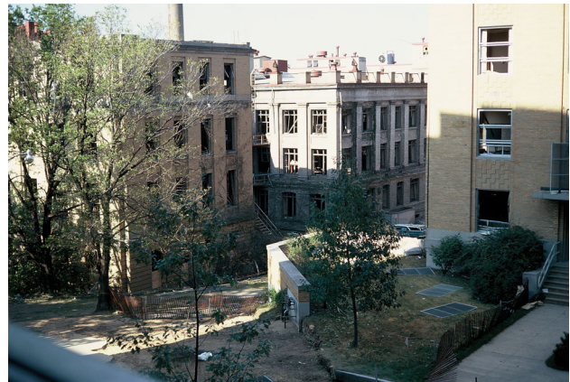
Fig. 4 Devastation of the Departments of Botany (right) and Mathematics (left), University of Wisconsin, Madison, USA, August 24th 1970
