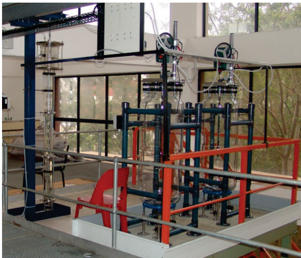
Pilot plant unit for recovery of luminophores
