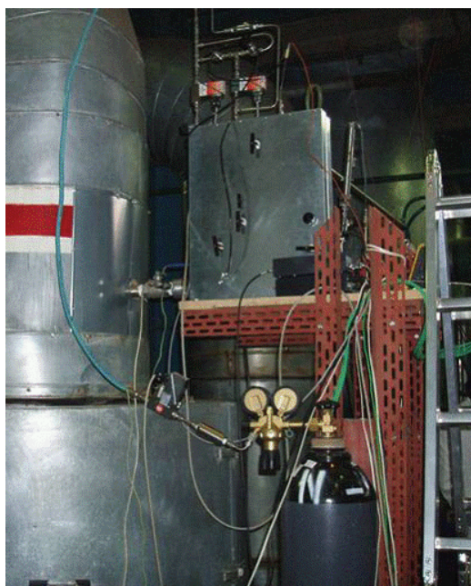
Aerosol sampling train connected to the turbine at thermal power plant Pruněřov II
