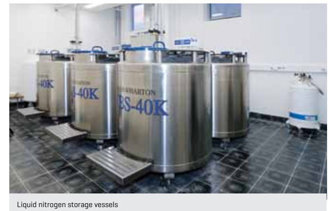
Liquid nitrogen storage vessels
