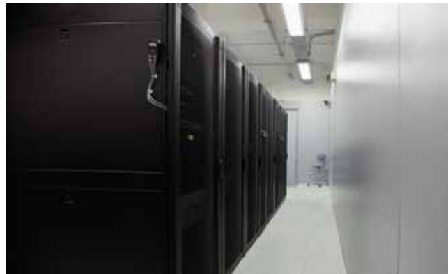
Main data centre room
