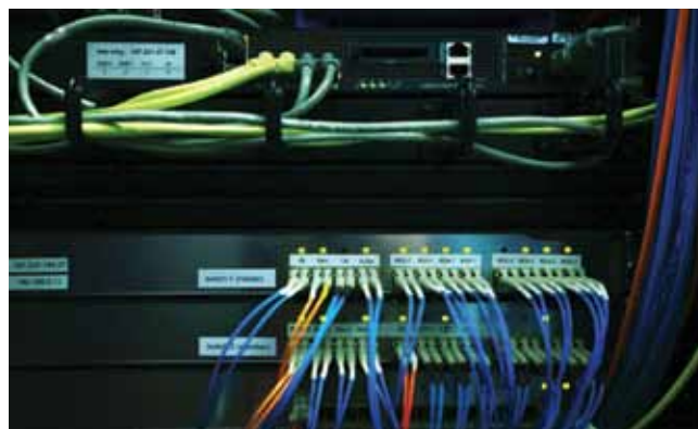
Firewall and central switch
