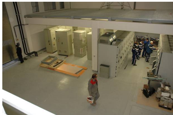
Fig 2.9: Assembly hall and power supply area.
