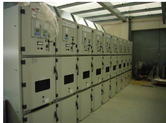
Fig. 3.7: High-voltage area – part of the 6kV switching station.
