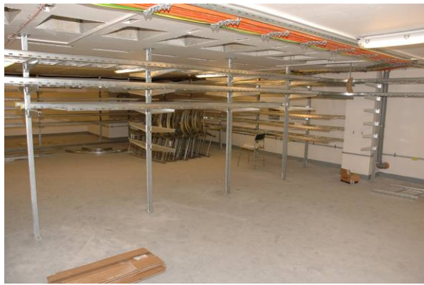
Fig 2.7: Cabel compartment – direction to flywheel generators .
