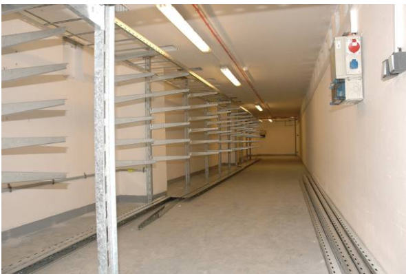
Fig 2.8: Cabel compartment – direction to transformers and convertors.
