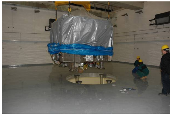
Fig. 1.7: The COMPASS tokamak is placed on its final location in the new tokamak hall.
