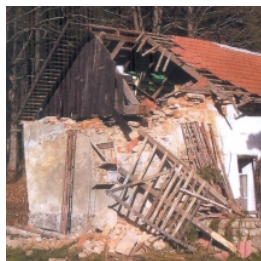
A house damaged by a fallen tree.
