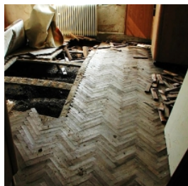
Buckling of a wooden floor structure.
