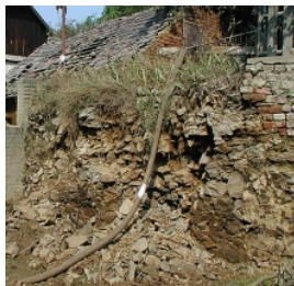
A destroyed stone-masonry retaining wall constructed with clay mortar.
