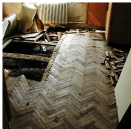
Buckling of a wooden floor structure.
