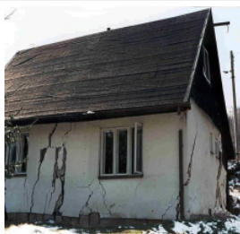
A house with cracks due to displacement.
