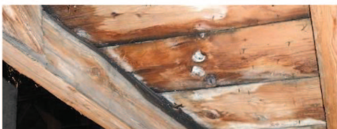
Figure 3: Lower part of the rafter damaged by wet rot
