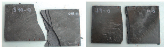
Figure 4: Aspect of the fracture of a slate samples collected from the roof after tensile testing – North plane sample with visible delamination (left), South plane sample (right)
