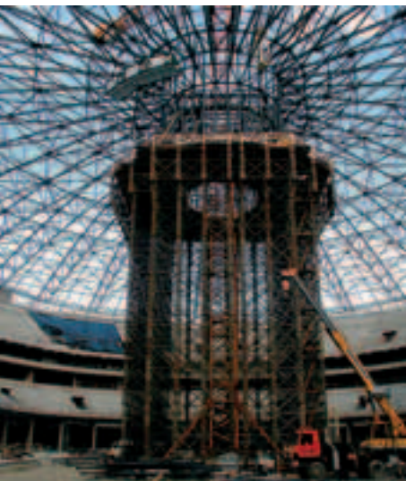
Steel roof structure of the Sazka hall, whose stress state was verified by experiment at the Institute of Theoretical and Applied Mechanics
