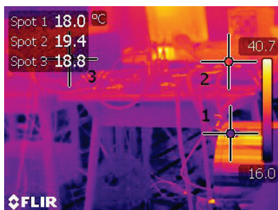
Fig. 2: Images taken by FLIR infrared camera
