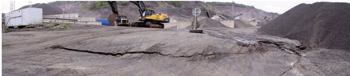
Fig. 3: Open cracks at the offices of the quarry Dobkovičky on the day before landslide
