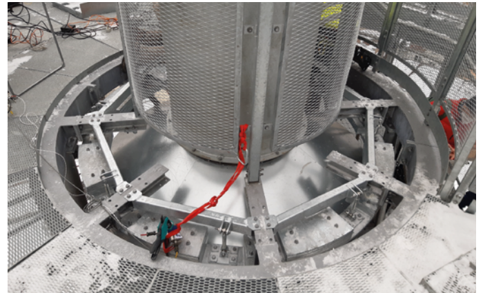
Fig. 2. Ring absorber with sensors already deployed. Photo: S. Hračov
