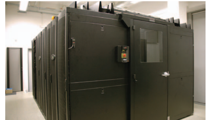
Main data centre room
