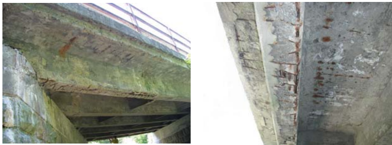
Fig. 1: Diagnosed bridges in villages Kolárovice and Topolčianky.
