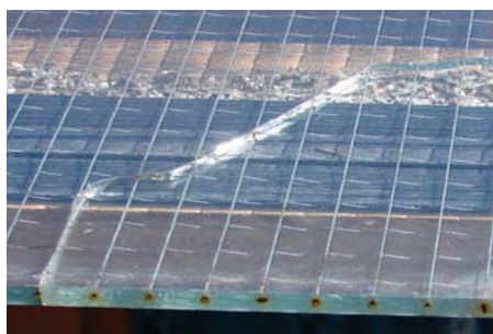
Fig. 4: Fracture due to corrosion of wires
