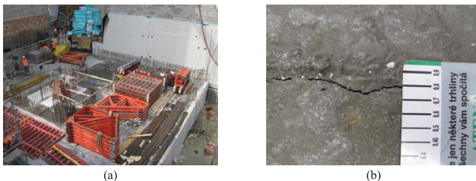
Fig. 1: Foundation block of a residential building in Prague, Czech Republic: (a) construction side overall view and (b) detail of 0.8mm crack width caused by concrete shrinkage.
