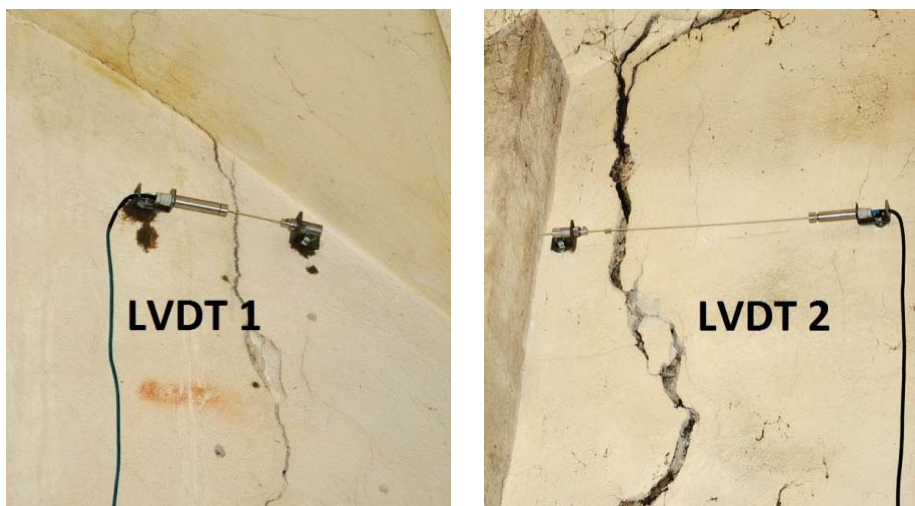
Fig. 10: LVDT set up, a) an inner side of the wall, b) an exterior side of the load-bearing wall
