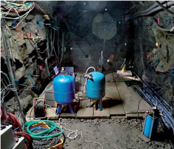
■ Fig. 14. View of the Josef gallery, JP47 site, in the course of a tracing test. Tracer solutions, present in the blue tanks, are pumped into the fracture through a steel tubing. The tested fracture system is located in the right corner above the floor (photo by J. Rohovec).
