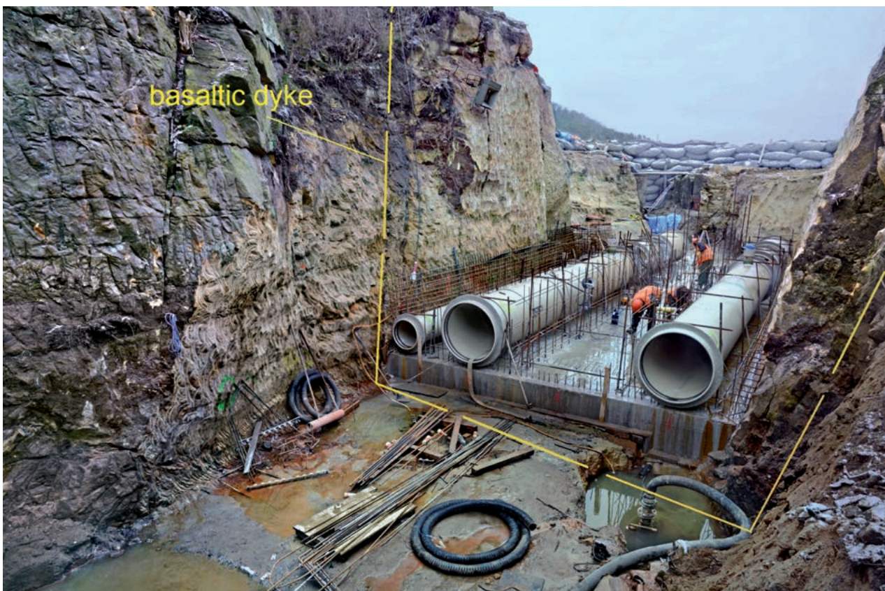
■ Fig. 18. Reconstruction of the outflow sluice in the dam of the Máchovo jezero Reservoir in January 2015. The newly discovered basaltic dyke, totally argillized, is highlighted in yellow (photo by J. Adamovič).
