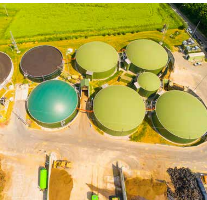
Equipment for biogas purification
