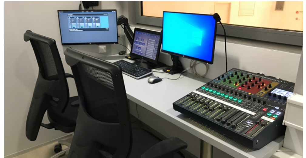
Audio video control room in the Conference hall
