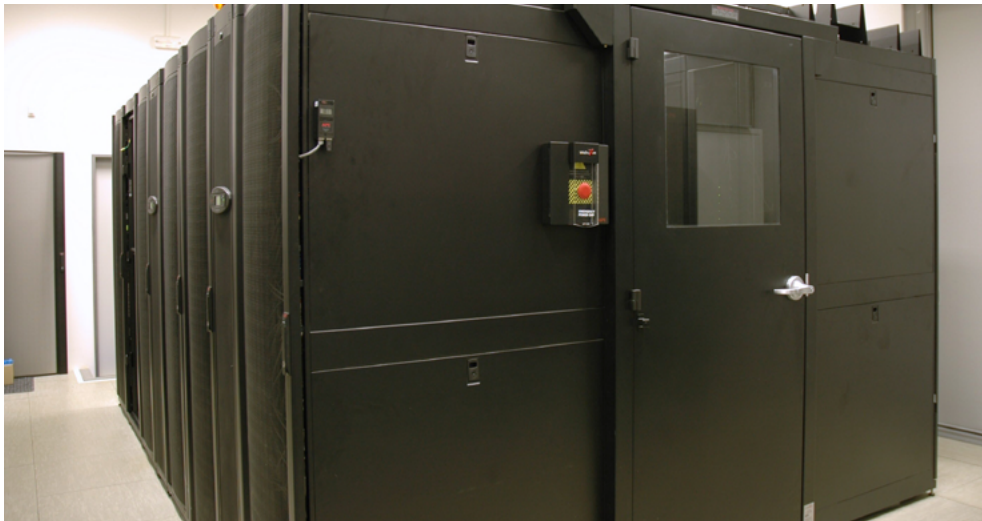
Main data centre room
