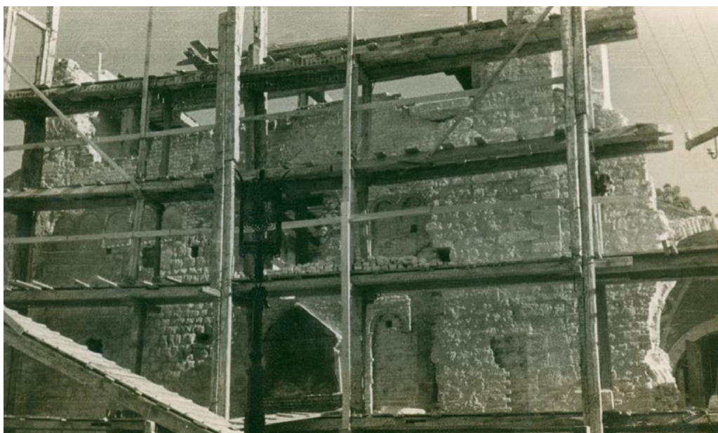
⬆ Fig. 8. Façade of the Senj Cathedral during reconstruction, August 1947 (photo Tihomil Stahuljak, Ministry of Culture and Media, Directorate for the Protection of Cultural Heritage, Photo Archive, Inv. Nr. 5063)
