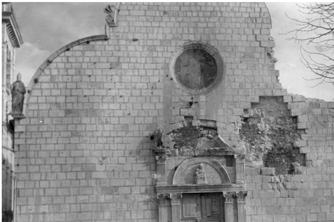
↑ Fig. 9. Damaged façade of the Osor Cathedral, prior to restoration, 1953 (photo Kocijančić, Ministry of Culture and Media, Archive of the Conservation Office in Rijeka, Inv. Nr. 3897-I-1250-Osor 67)
