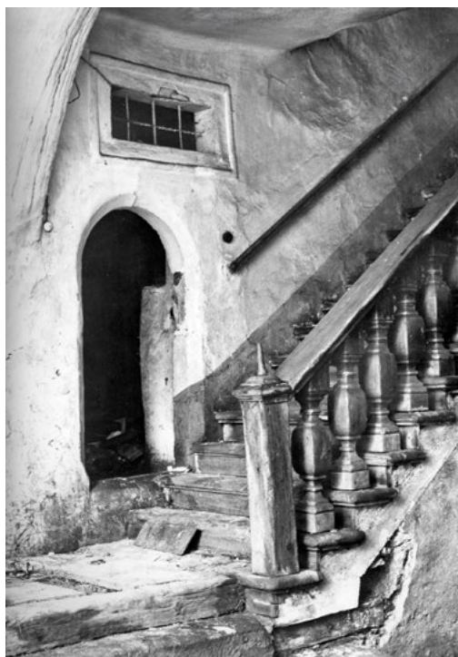
⬆ Fig. 13. Rožmberk nad Vltavou, interior of the staircase of the townhouse no. 76 with visible medieval constructions, on the reverse side is a record of the photo taken five hours before the collapse of the building, 18 April 1962 (photo Petr Pešek, photoarchive of the National Heritage Institute, Regional Office in České Budějovice)
