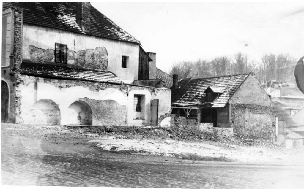
⬆ Fig. 10. Týn nad Vltavou, demolition of townhouses within reach of the rising river level, 1962 (Photoarchive of the National Heritage Institute, Regional Office in České Budějovice)
