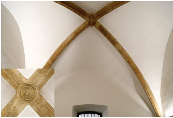
Fig. 110. Brno, 2 Minoritská Street. Vaulted chamber ('kamenate') with a keystone. Photo by M. Peška.
