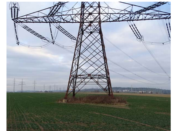
Electricity pylons are overlooked refuges for small mammals in agricultural landscapes. | Photo by M. Šálek
