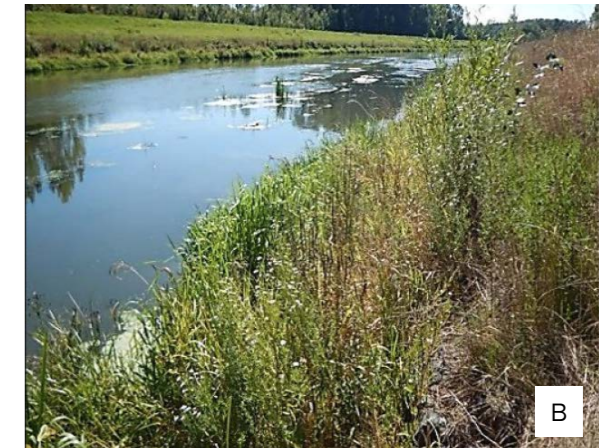
A) Banks of the River Dyje in 2011, with rip-rap clearly visible; B) banks of the River Dyje in 2017, with rip-rap covered in a thick layer of sediment and aquatic/riparian vegetation. | Photos by L. Šlapanský
