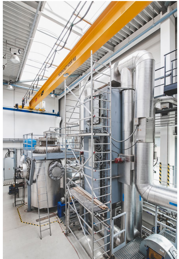
Fig. 5: Large LOCA vessel (on the left) and the air overheater for heating duplicated shells of vessels (on the right)
