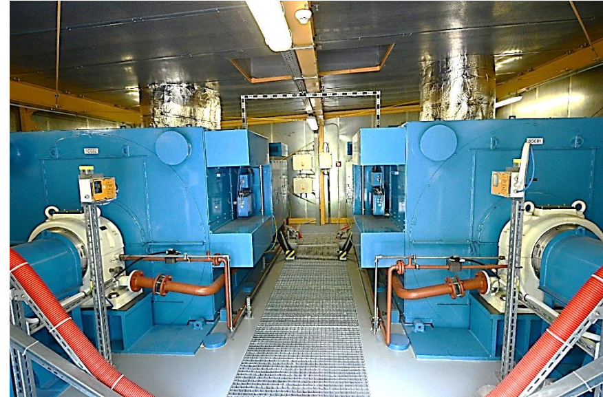
COMPASS fly-wheel generators
